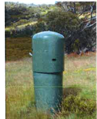
Figure 4: Photo of a hydrant.
